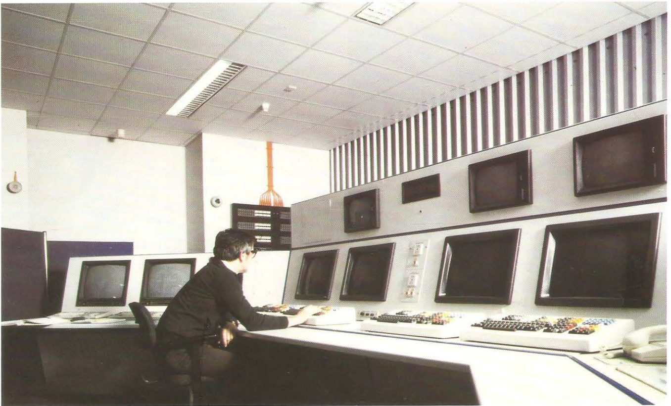
General view of the control room. The signalling control screens and keyboards are in front of the operator, the power control screens (SCADA) are on his left side and the closed circuit television (CCTV) monitors are on the upper part of the desk. The master time clock is in the centre of the desk.
