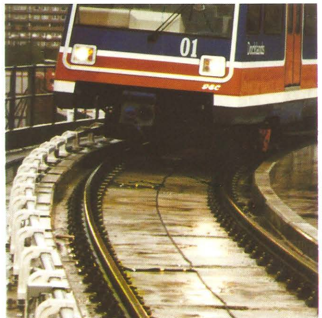
The signal cables transpositions are closely spaced here to provide a low speed around the sharp curve.
