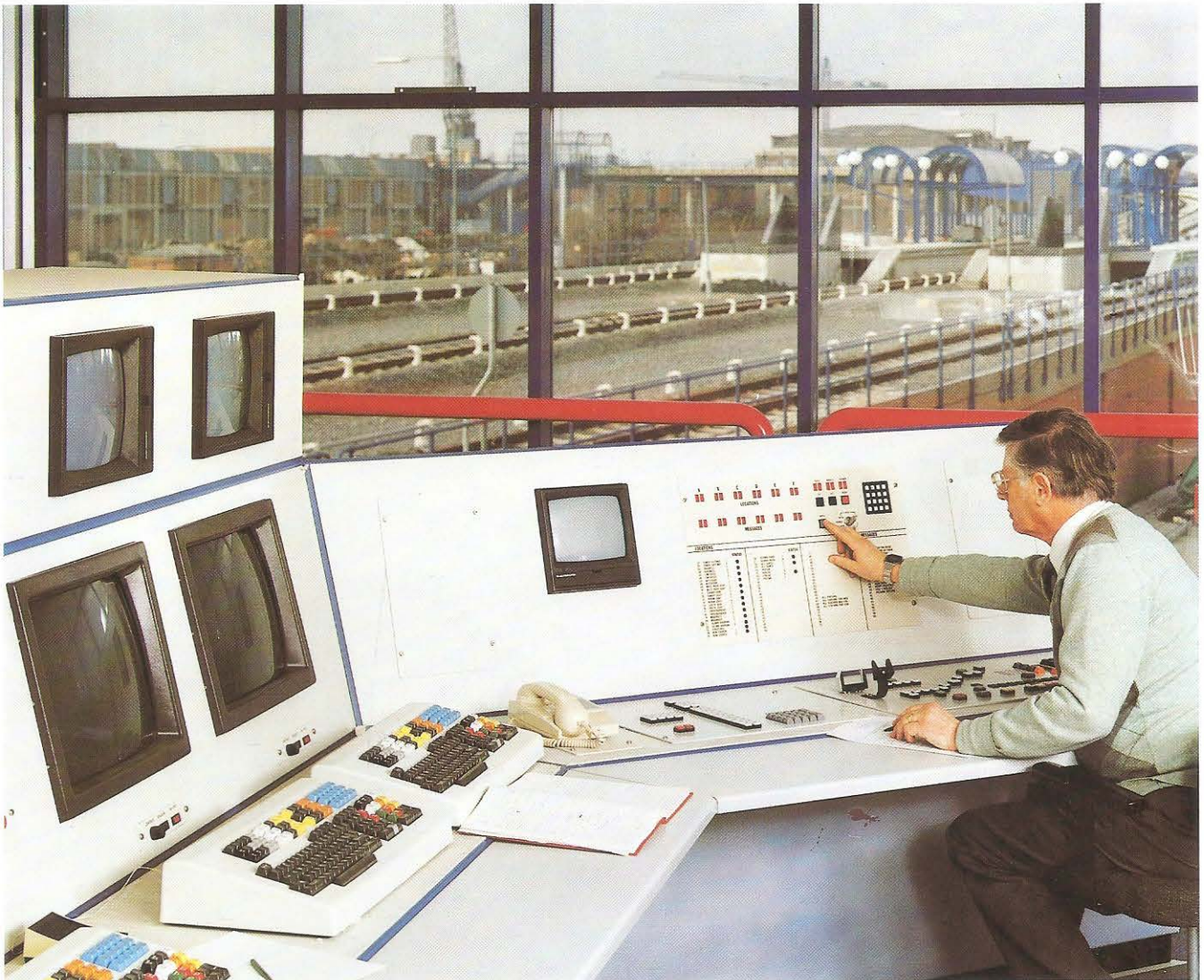
Poplar station from the controllers' desk in the control room showing the passenger alarms, CCTV monitors and public address controls on the desk.
