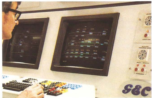
Close-up of the signalling controller's vdu screens.
